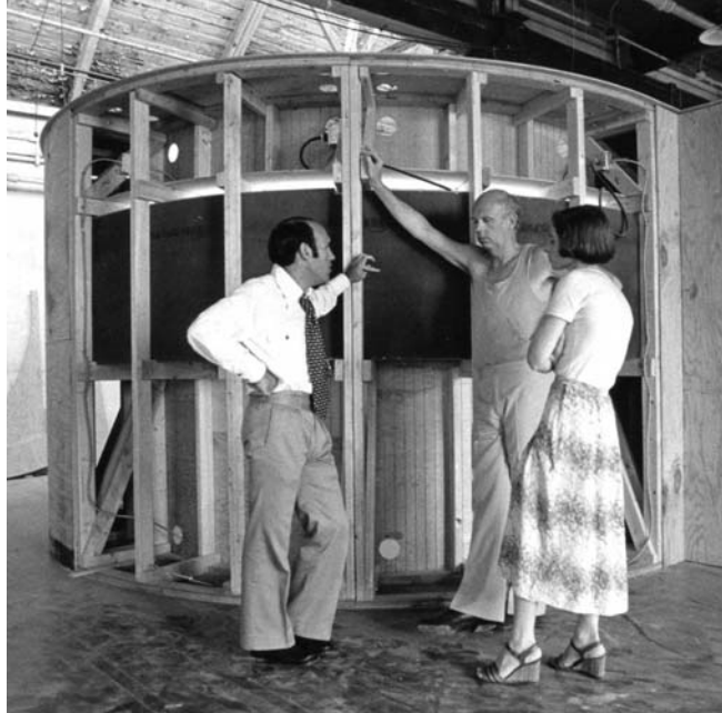
Stuart Cohen, Claus Oldenburg, and Judith Kirshner with Mouse Museum under Construction. 1977.
